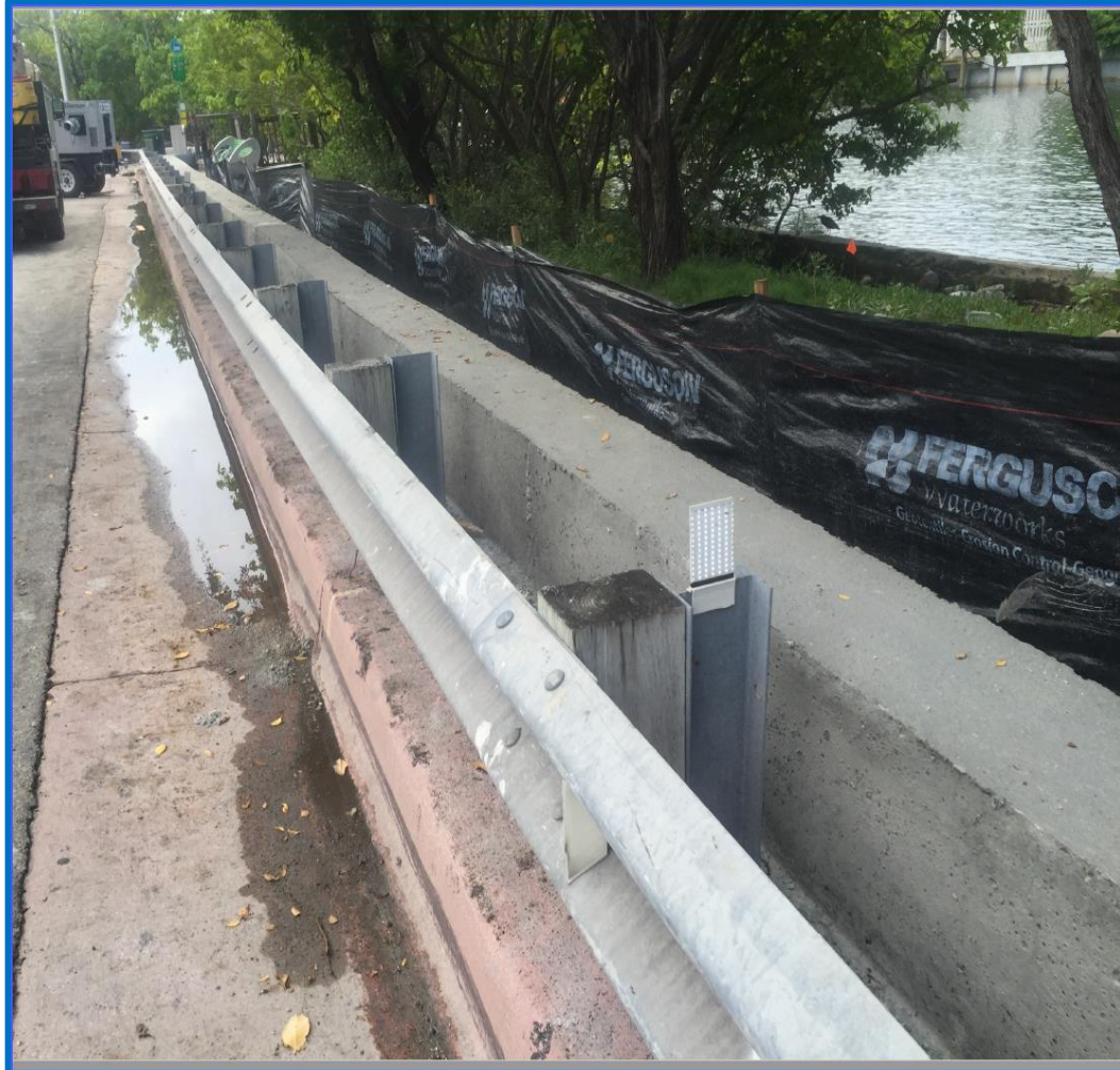
Figure #8. Photograph shows “temporary” concrete flood barrier built in early 2016 along Indian Creek Drive that reduced the risk of flooding from water overtopping the seawall.
