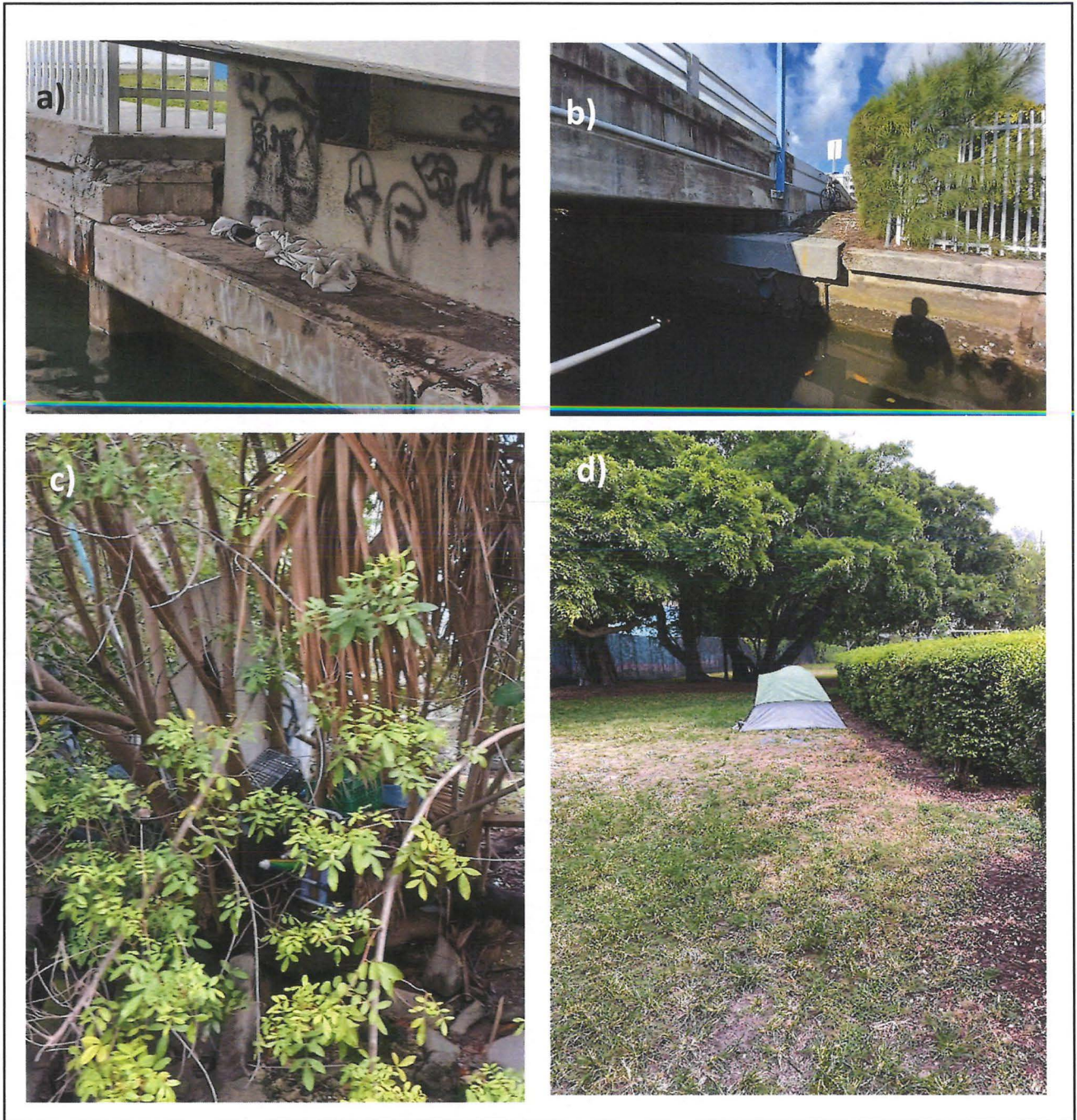
Figure D.8: Pictures of homeless encampments that were found immediately adjacent to the PVC. These encampments were located: a) underneath the bridge from PVI to Biscayne Shores Elementary School, b) bridge from PVI to Dickens Ave, c) mangroves in the vicinity of the park adjacent to the PVC Kayak Launch, and d) immediately west of the community garden area adjacent to Park View Island park.
